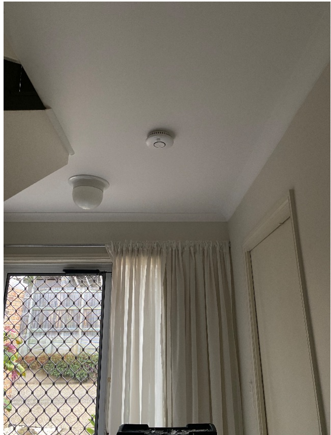
Essentials Smoke Alarm Service - 3
