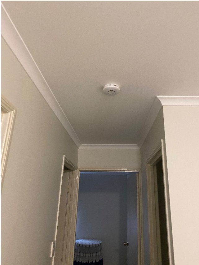
Essentials Smoke Alarm Service - 4
