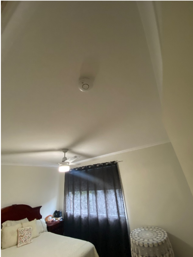
Essentials Smoke Alarm Service - 1
