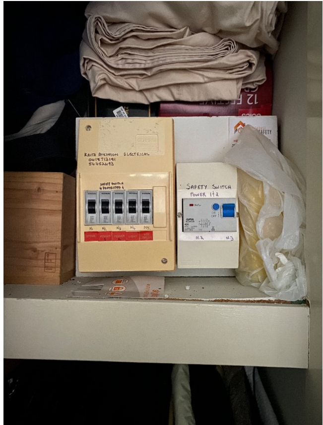
Essentials Safety Switch Testing - 1
