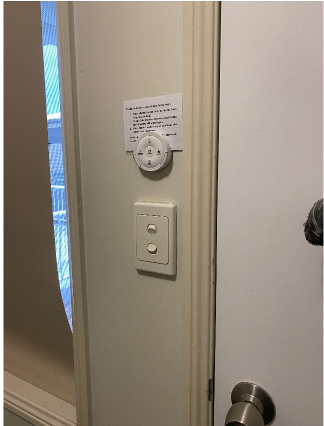
Essentials Smoke Alarm Service - 1
