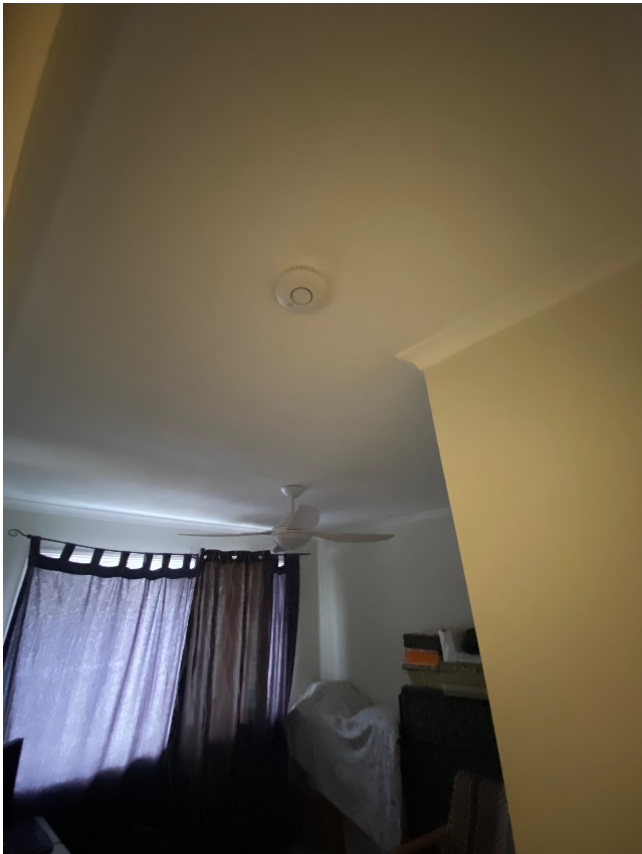
Essentials Smoke Alarm Service - 2
